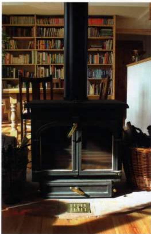
Above left: Clearview wood burner provides back-up heating.
